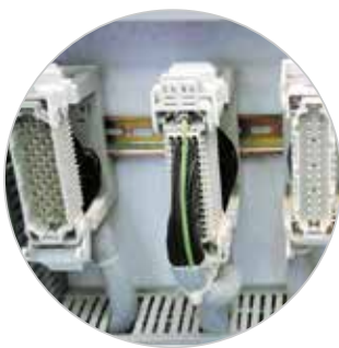
Cabinet mounted with rail cases
